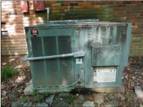
8.7 Item 1(Picture) HVAC System
