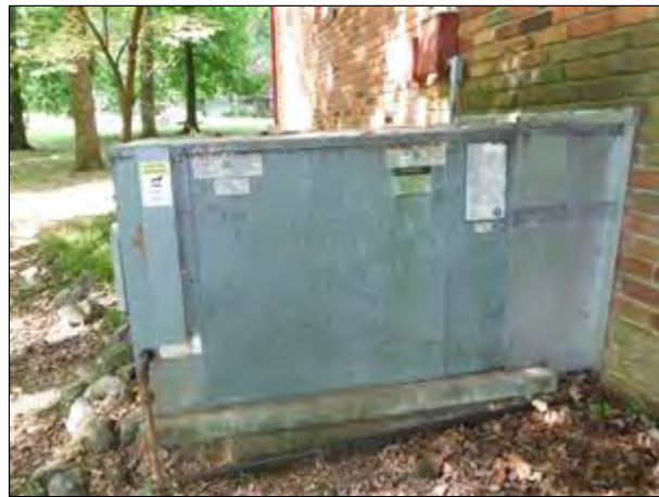
8.7 Item 4(Picture) HVAC System
