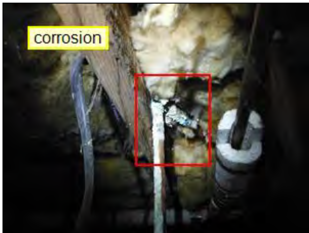
6.1 Item 11(Picture) Water Line above water heater
