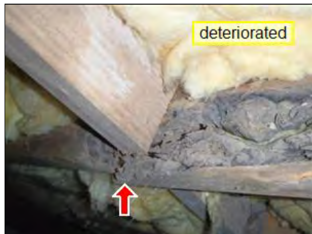
5.3 Item 4(Picture) Joist under front bedroom
