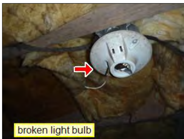
7.3 Item 3(Picture) Light in crawlspace
