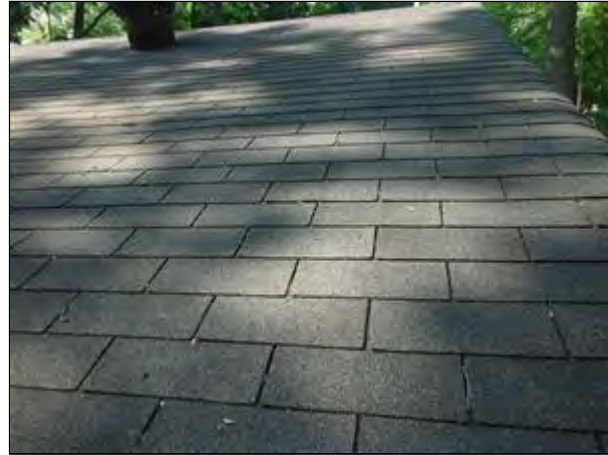
1.0 Item 2(Picture) Shingles
