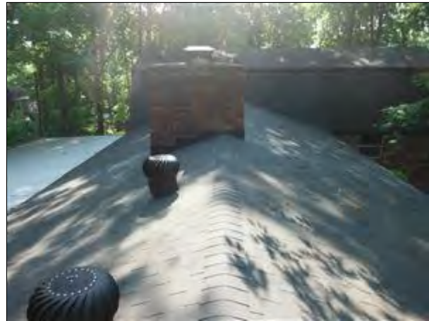
1.0 Item 4(Picture) Shingles
