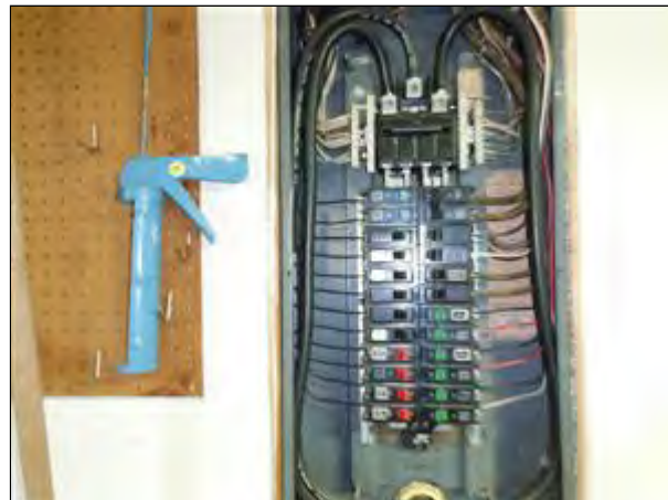
7.6 Item 2(Picture) Electrical Panel
