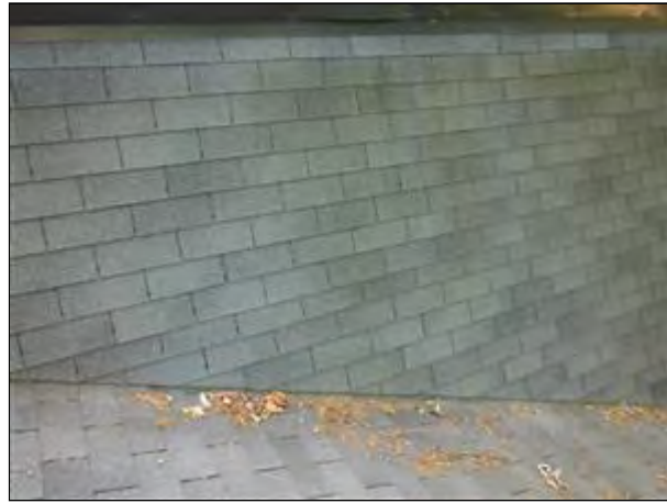
1.0 Item 6(Picture) Shingles
