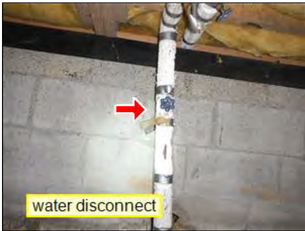
6.3 Item 1(Picture) Water shut off under home
