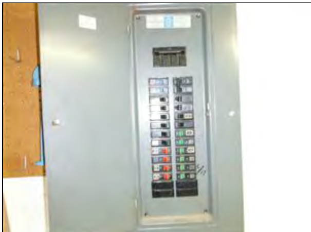
7.6 Item 1(Picture) Electrical Panel
