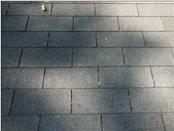
1.0 Item 3(Picture) Shingles
