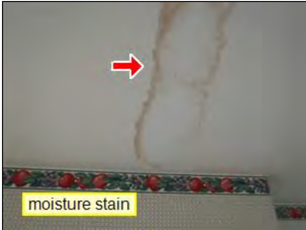
4.0 Item 1(Picture) Kitchen Ceiling
