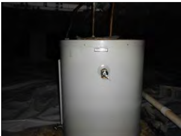
6.2 Item 1(Picture) Water Heater
