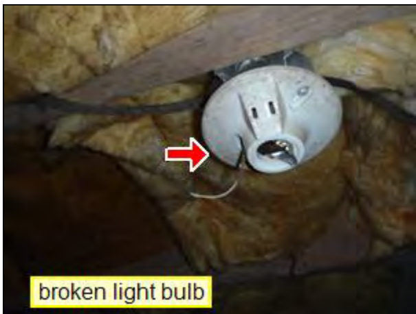
7.3 Item 3(Picture) Light in crawlspace
