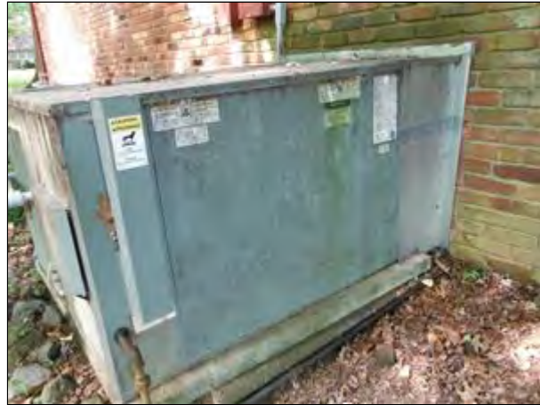
8.7 Item 2(Picture) HVAC System
