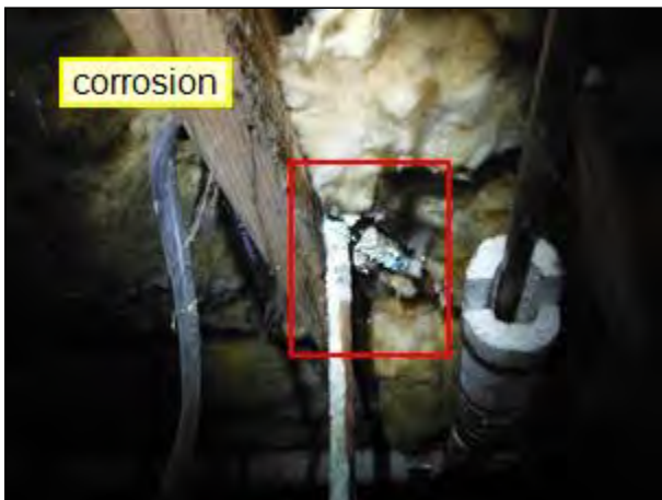
6.1 Item 11(Picture) Water Line above water heater
