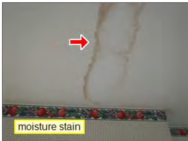
4.0 Item 1(Picture) Kitchen Ceiling
