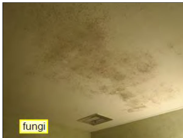
4.0 Item 2(Picture) Master Bathroom Ceiling
