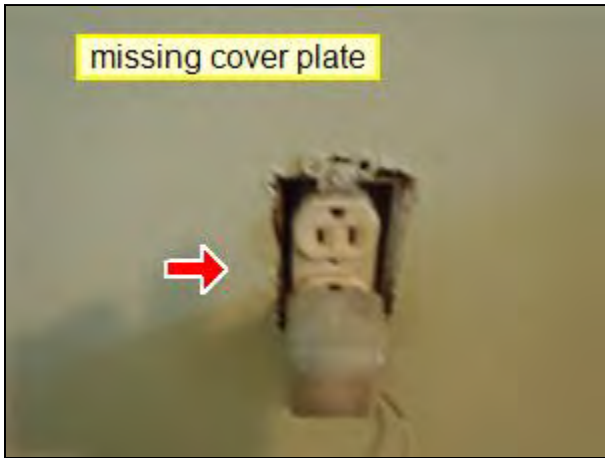
7.3 Item 1(Picture) Outlet upstairs
