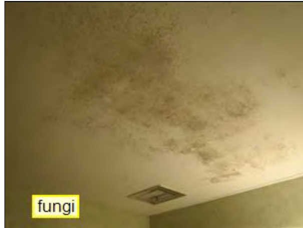
4.0 Item 2(Picture) Master Bathroom Ceiling
