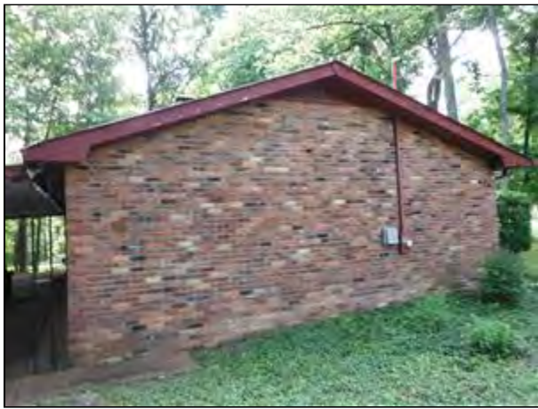
2.0 Item 1(Picture) Left side of home
