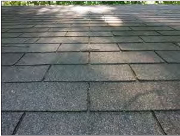
1.0 Item 5(Picture) Shingles
