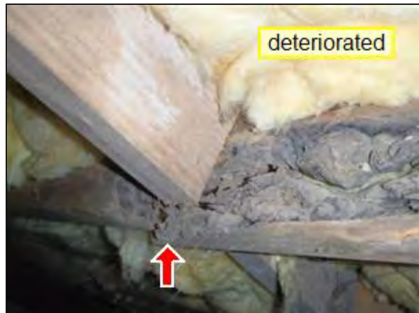
5.3 Item 4(Picture) Joist under front bedroom
