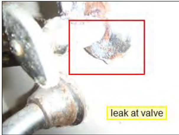
6.1 Item 10(Picture) Laundry room sink
