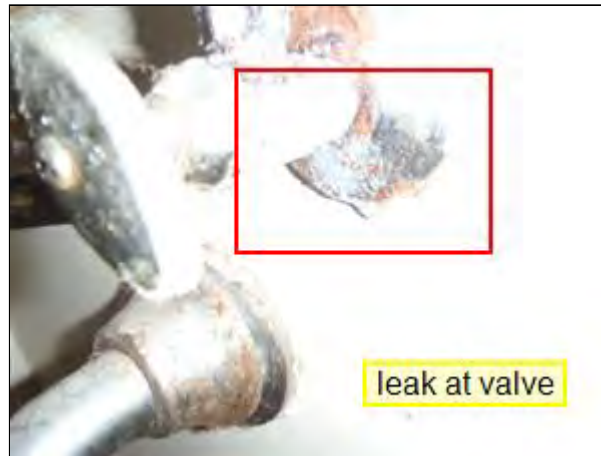
6.1 Item 10(Picture) Laundry room sink
