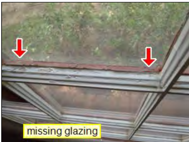
4.6 Item 1(Picture) Front right bedroom
