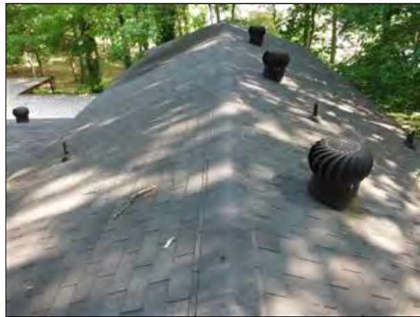
1.0 Item 8(Picture) shingles
