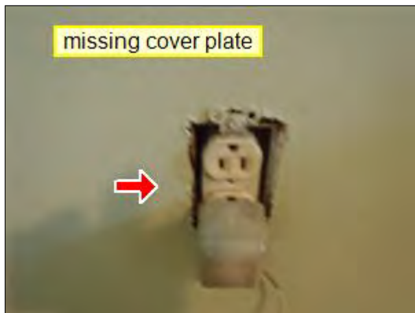
7.3 Item 1(Picture) Outlet upstairs
